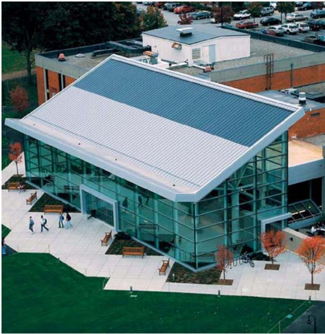
■ Building integrated photovoltaics were installed on the roof of the Slavin Center. Photo by John Scott, AIA, Symmes Maini & McKee Associates Inc.
